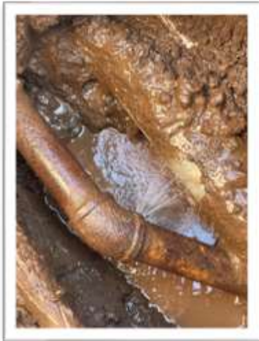
The leak, with water barely turned on
