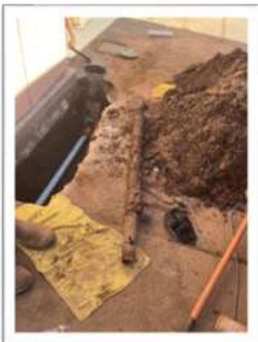
A new, larger leak was repaired about five feet away from the original, smaller leak
